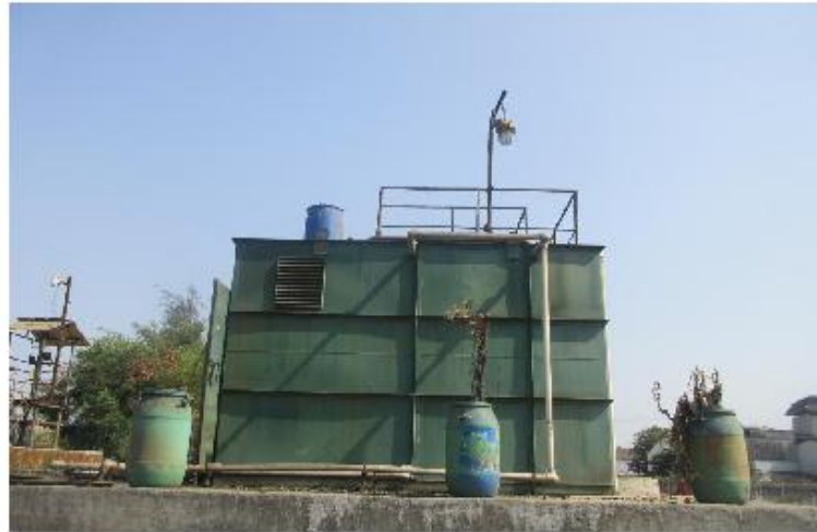
Annexure No.-3- Sewage Treatment Plant
