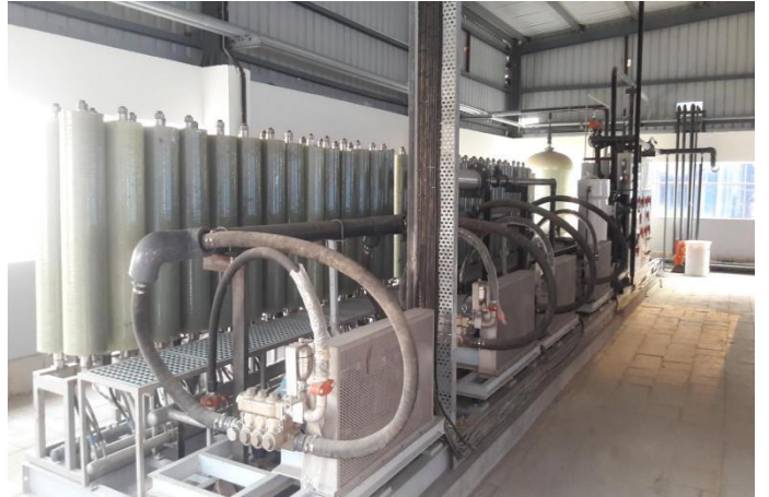
Reverse Osmosis Plant
