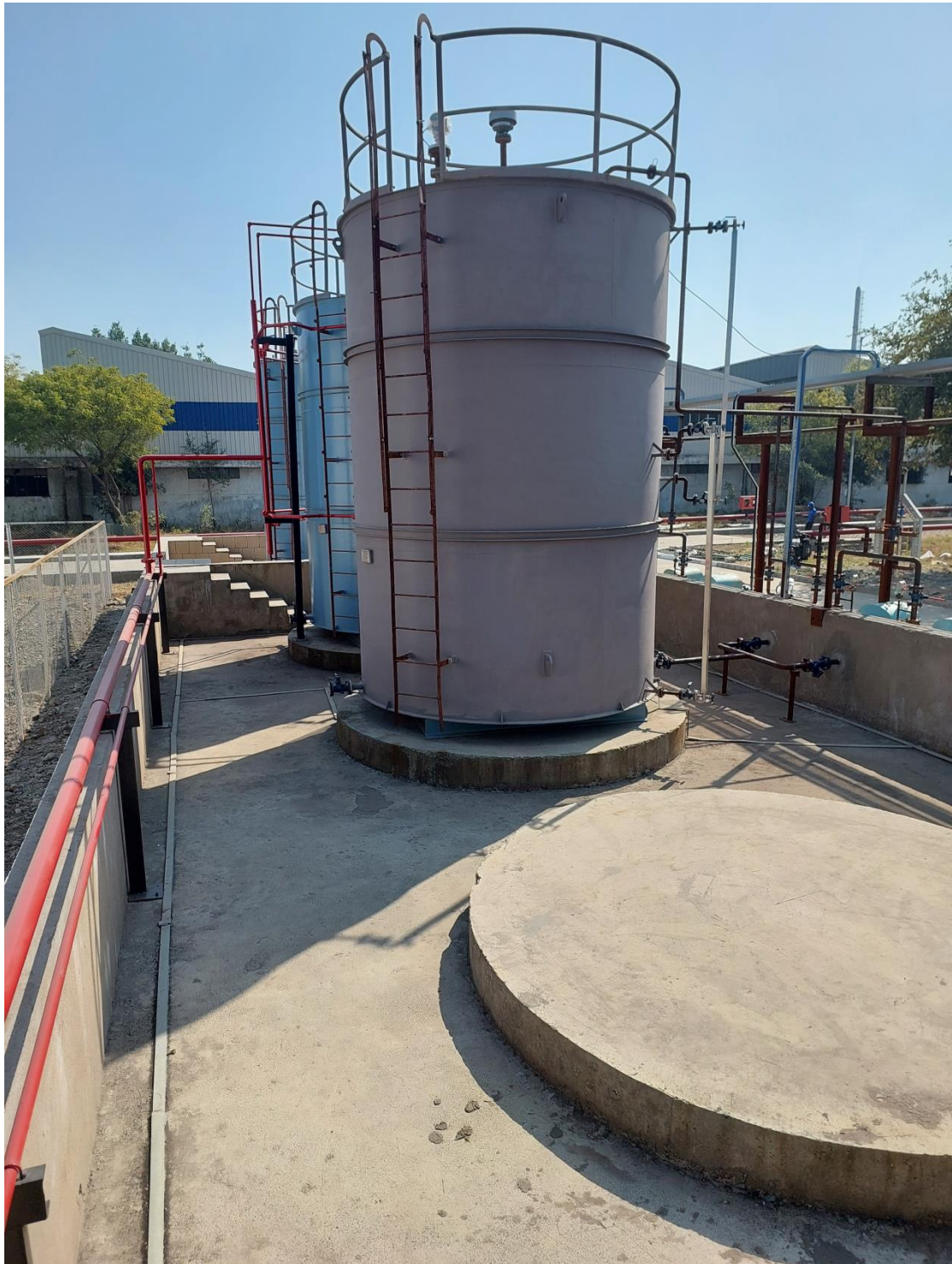
Dyke wall of Chemical Storage Tank
