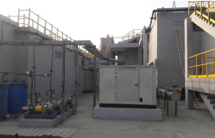
Effluent Treatment Plant
