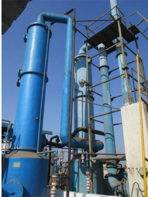
1. Block-1 Process Stack (S-2):
